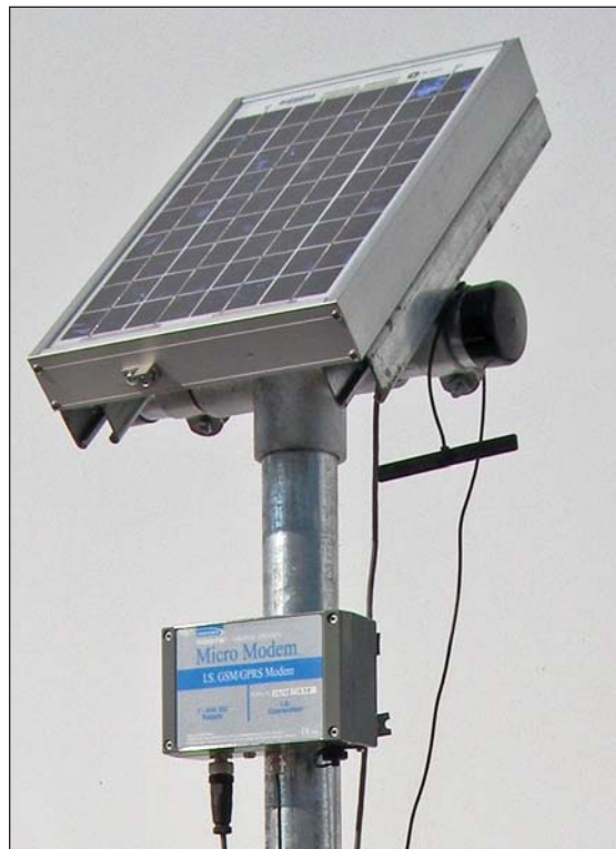
GSM/GPRS Modem installation complete with solar panel.
