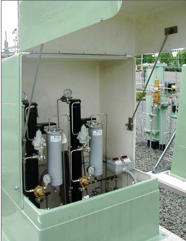
Figure 7.0 - Dual PICs Installed in Becker CAB Series Fiberglass Enclosure Two Becker PIC Pressure Instrumentation Columns are installed inside a Becker CAB Fiberglass Cabinet. Each PIC provides conditioned and regulated supply gas to a Becker control valve, one PIC for the working control and one PIC for the monitor control valve. Each PIC also includes the optional Becker FD-1500 Filter-Dryer to remove moisture from the supply gas. The fiberglass enclosure is required to prevent the catalytic heaters from extinguishing during inclement weather. Each catalytic face heater is hard wired with 120 V A.C. starting voltage and each disconnect is also located inside the fiberglass enclosure.
