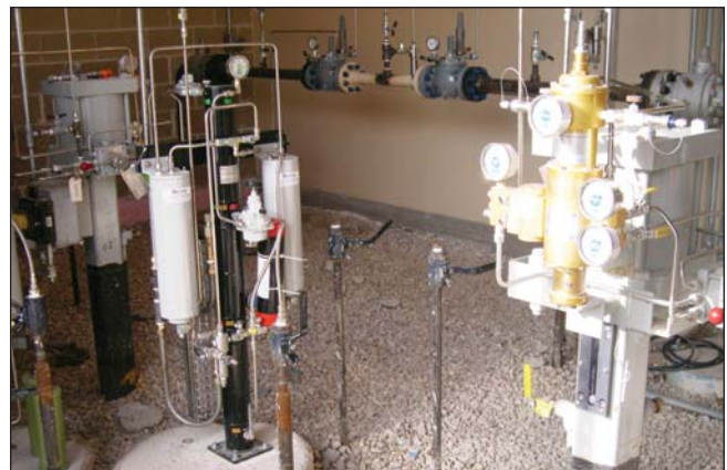
Figure 2.0 - PIC Installed Inside Natural Gas Regulation Facility
