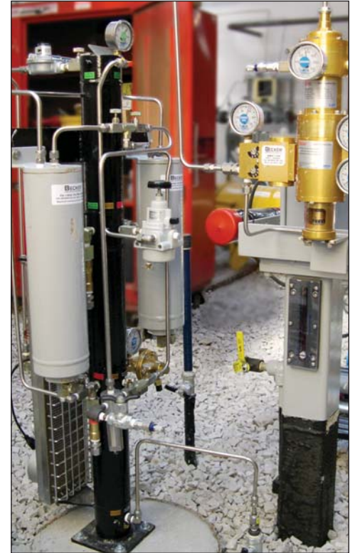
Figure 9.0 - PIC Installed Inside Pressure Limiting Station Building
