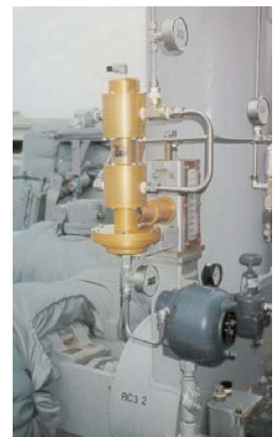
Figure 8.0 - Surge Control Valve
