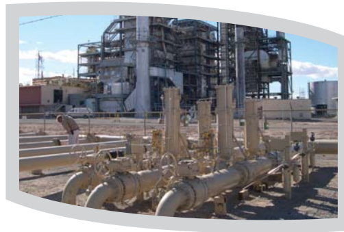
Figure 12 - Slam Shut and Fast-Acting Monitor Regulators Natural Gas Fired Power Plants (Power Generation Industry) Fast-Acting Monitor Regulators and Slam Shut Valves provide the ultimate protection to Natural Gas Fired Turbines from overpressure occurrence. These monitor regulators and slam shut valves utilize Surge Design RPSR Actuators to ensure quick stroking and minimize potential of damage to downstream pipe and equipment in the event of potential over-pressurization. Slam Shut shut valves and fast stroking monitor regulators are standard to most Becker pressure regulator stations that feed power plants due to their reliability and purpose built design.
