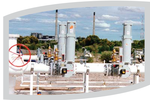
Figure 15 - Becker RPSR Actuated Control Valves in Power Plant
